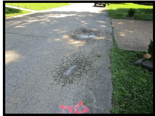
Garibaldi Place: Alligator Cracking w/ Potholes
