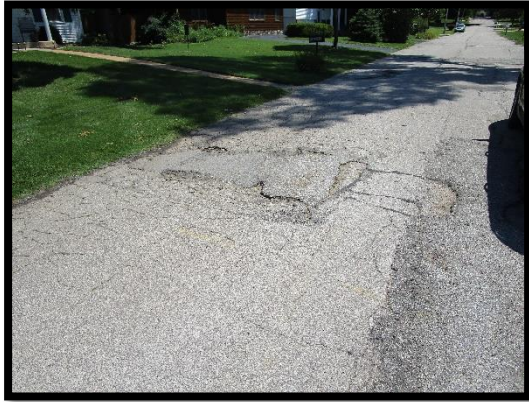
Arthur Place: Longitudinal & Transverse Cracking, Alligator Cracking, Raveling, & Potholes
