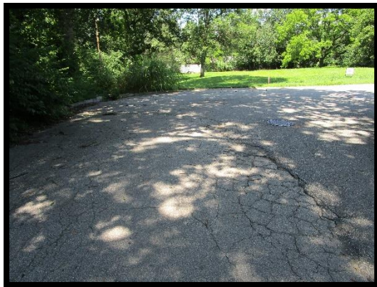
Princess Avenue: Longitudinal & Transverse Cracking, Alligator Cracking, & Raveling
