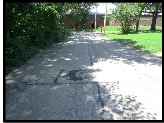
Cable Avenue: Longitudinal & Transverse Cracking, Alligator Cracking, Raveling, & Potholes
