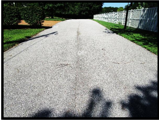
Donoho Place: Longitudinal & Transverse Cracking
