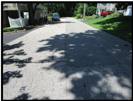
Savannah Avenue: Longitudinal & Transverse Cracking w/ Alligator Cracking
