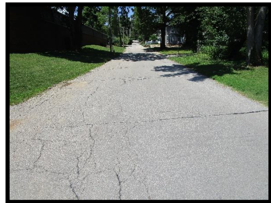
Dwyer Avenue: Transverse Cracking, Alligator Cracking, & Raveling
